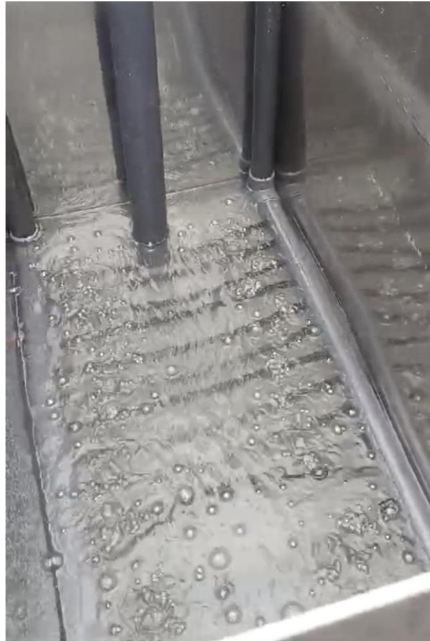
Aeration system implementation
