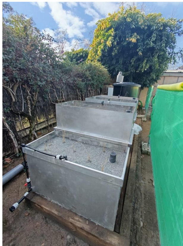
VSSF treatment wetlands
