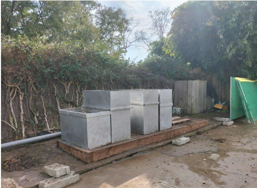
VSSF treatment wetlands
