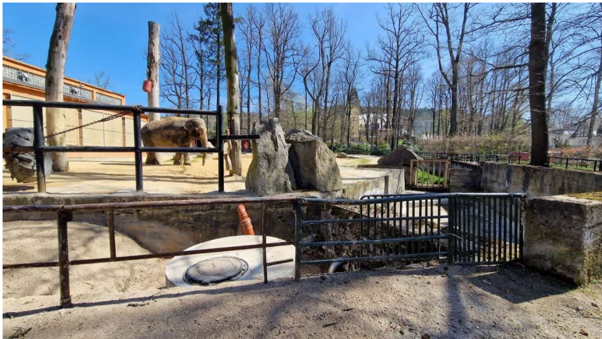
Connection of the outdoor elephant pool to the Watersave+ system.
