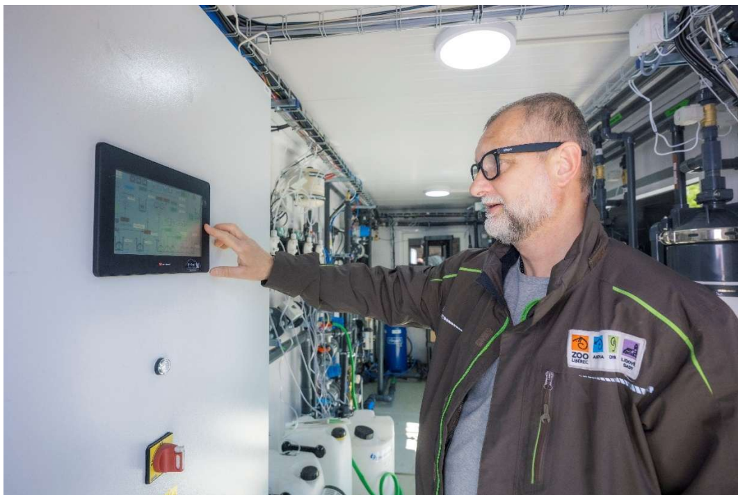
Measurement and control system
