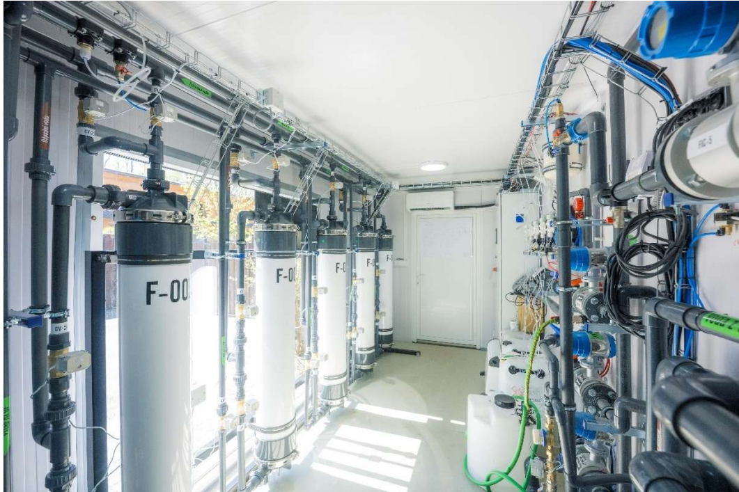
Water treatment plant unit with ultrafiltration
